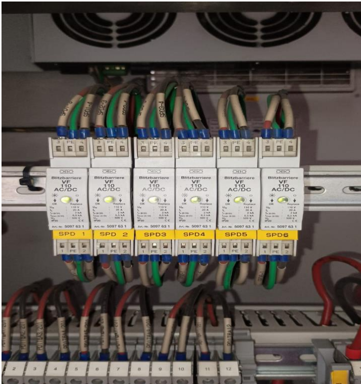
Fig. 2 Surge Protection Device Class D SPD 1,2,3,4,5,6 110V AC/110V DC
